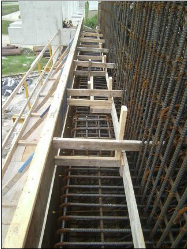
Timber Framing for a Pier Cap Note the chamfer strip along the left edge
